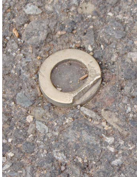
Figure J-6. A few circle markers were chipped by a front-end loader removing snow.
