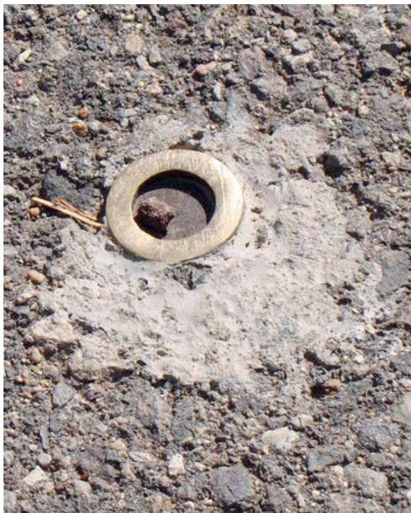
Figure J-4. Crumbled asphalt around some circle markers has already been patched.
