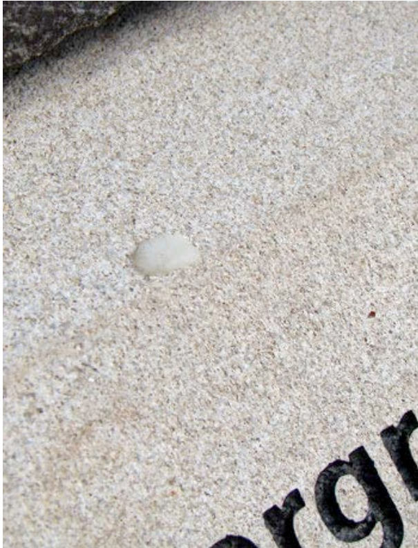
Figure J-13. Pine sap is dripping onto plinths in some places. This plinth has one drip.
